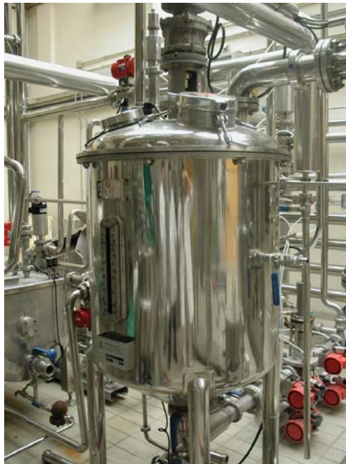
Picture 5. Deaeration tank (HRS)
